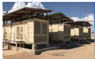
1700 KW Wartsila 20V34SG Natural Gas ...
