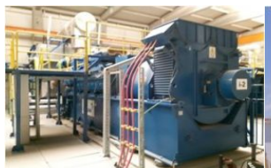
4000 KW Wartsila 20V34SG Natural Gas ...
