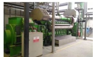
5000 KW Wartsila 20V34SG Natural Gas ...
