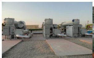
7500 KW Wartsila 20V34SG Natural Gas ...
